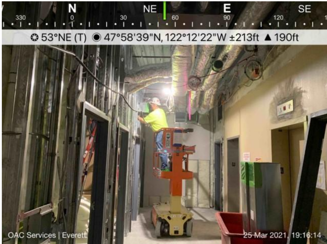
Lobby ductwork on Level 4.
