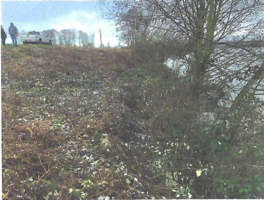
Photo D3: Sloughing landward of the trees on the riverward slope, downstream oriented (199+50).
