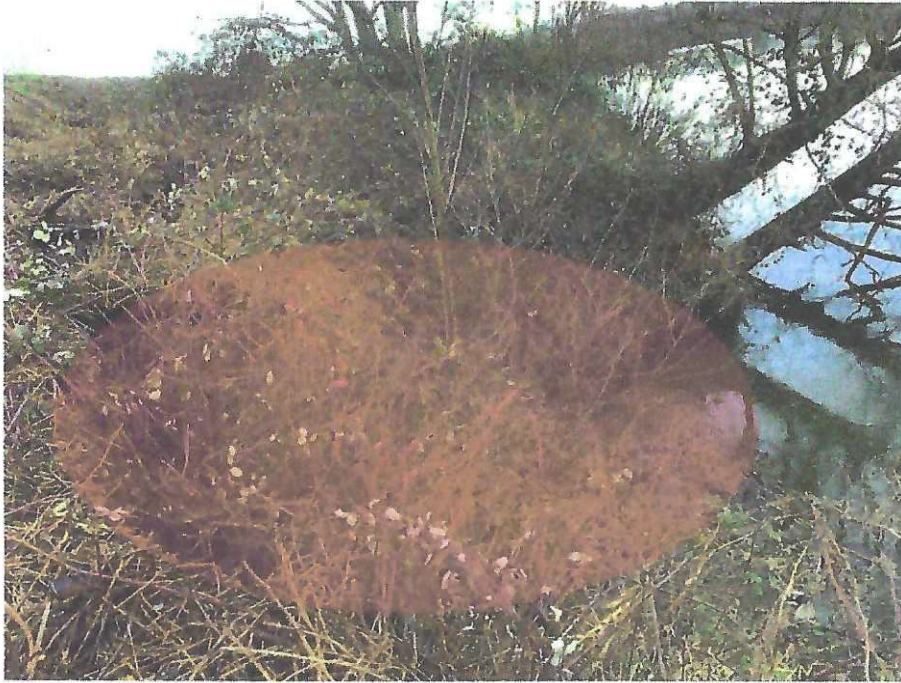
Photo D1: Riverbank Erosion, shown in red, downstream oriented (197+50).
