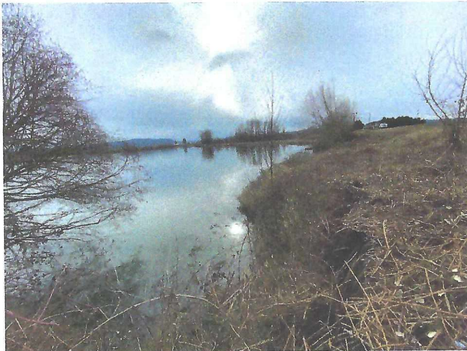
Photo D4: Scour hole and subsequent sloughing on the riverward slope, upstream oriented (STA 199+50).
