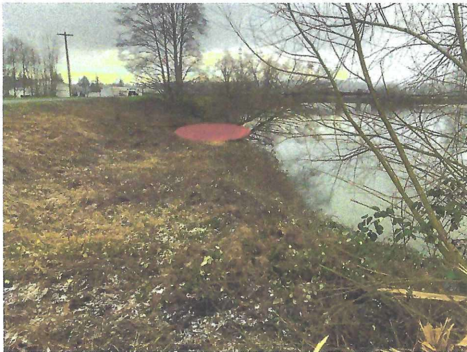
Photo D2: Scour hole, shown in red, on the riverward slope, downstream oriented (198+00).
