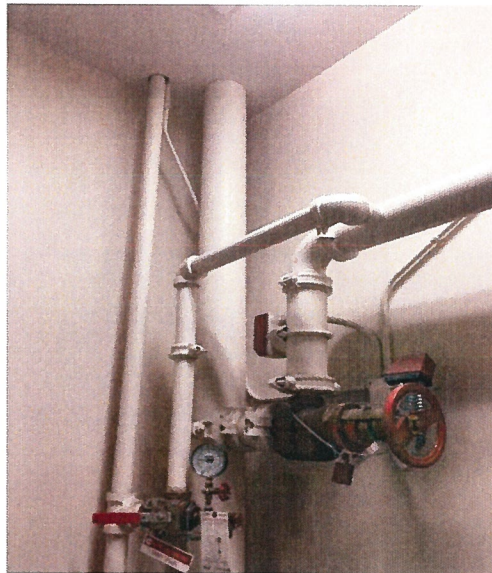
5 th Floor Stairwell Door - CR location & "New" Conduit pathway
