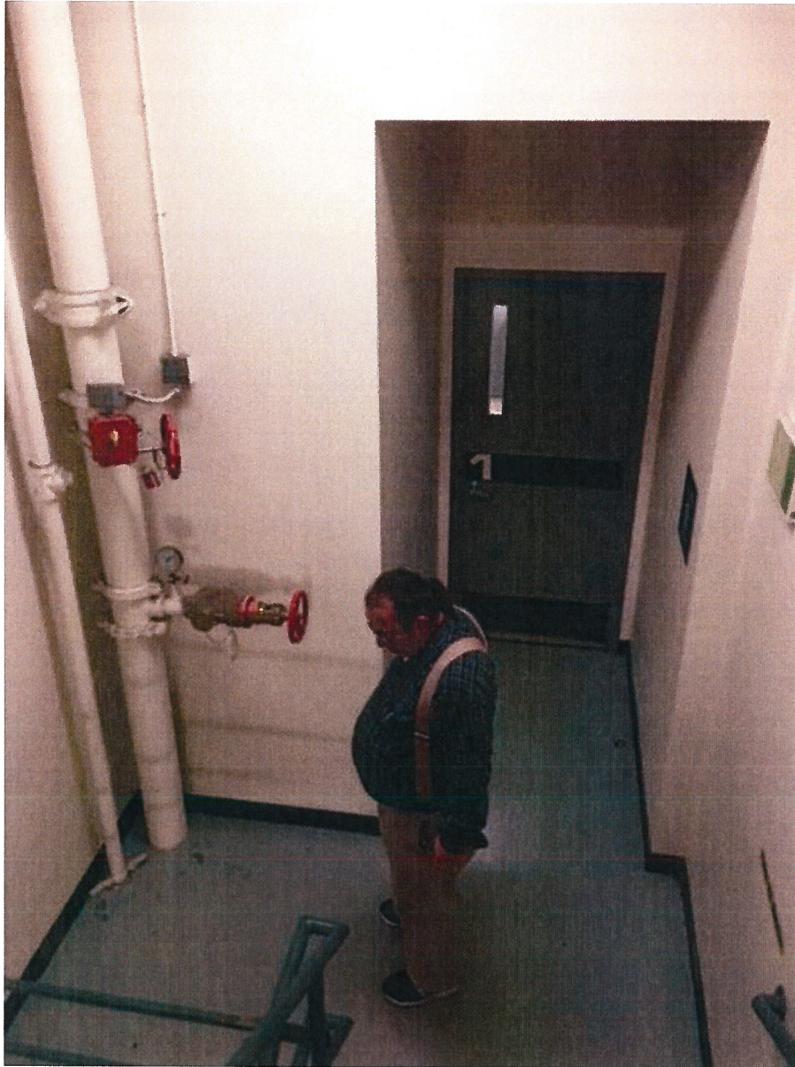
1 st Floor Stairwell Door – NO CARD READER ON THIS FLOOR. Continue conduit path to Basement
