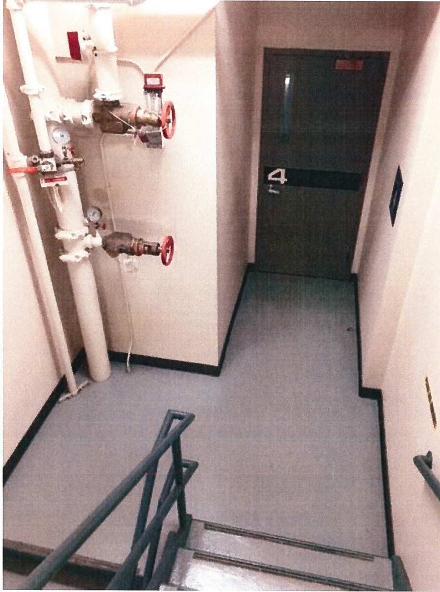
4 th Floor Stairwell Door - CR location & "New" Conduit pathway
