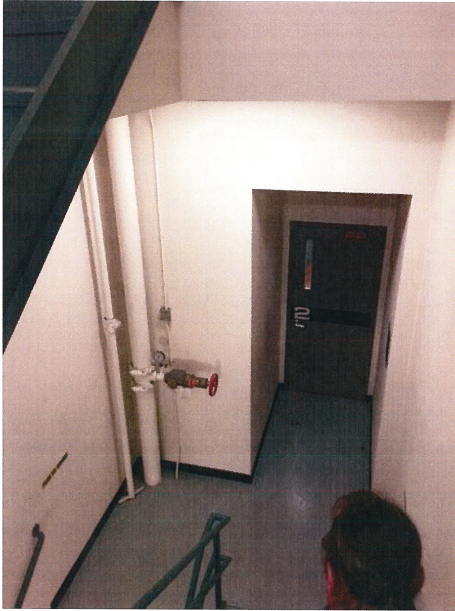
2 nd Floor Stairwell Door - CR location & "New" Conduit pathway
