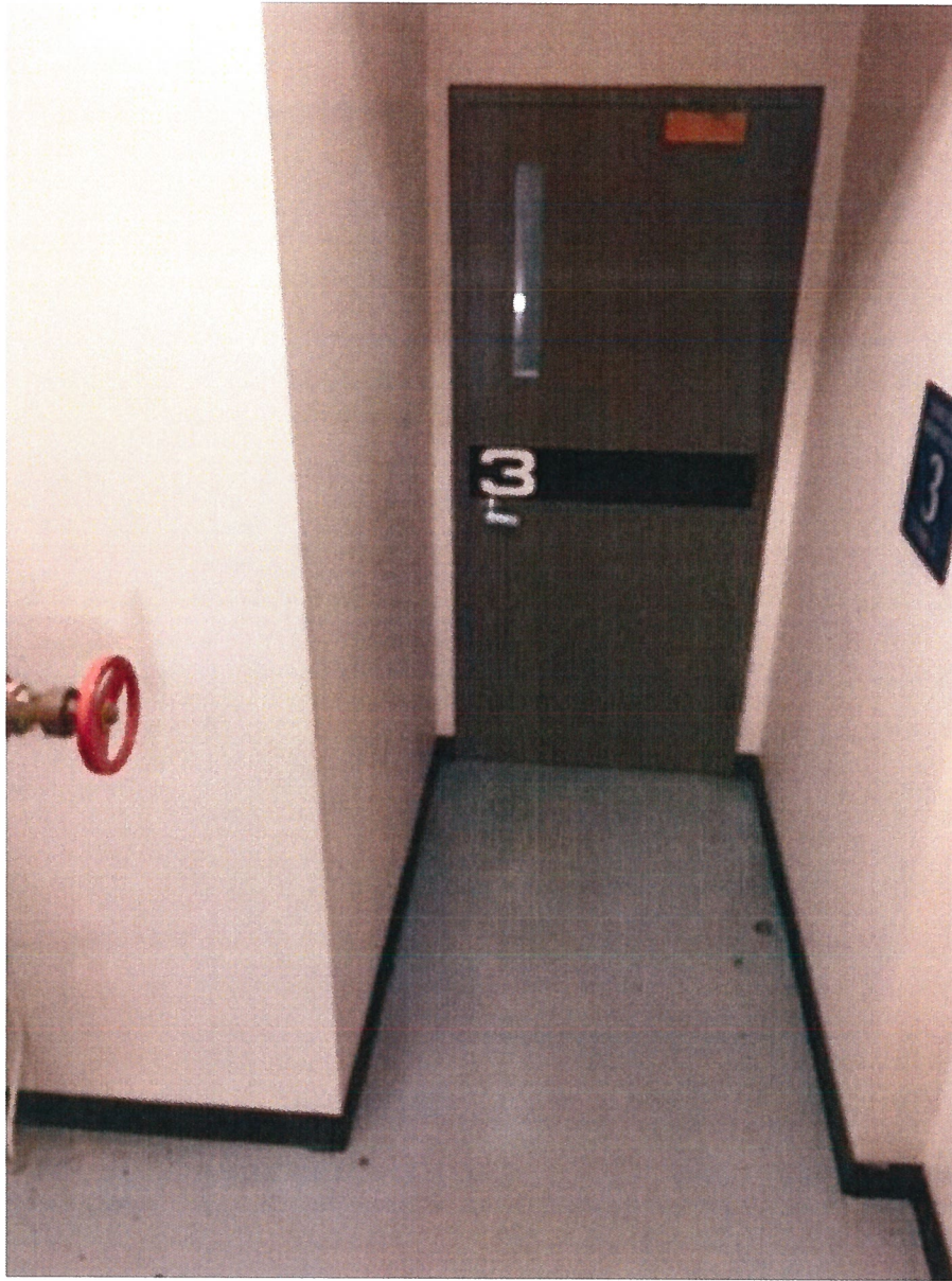
3 th Floor Stairwell Door - CR location & "New" Conduit pathway
