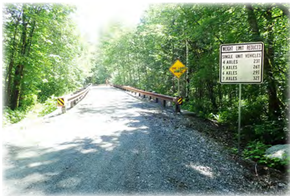
South Fork Sauk River Bridge 540 on Reece’s Hideout Road has a both a width and weight restriction.
