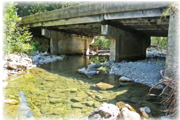
Coal Creek Bridge 556 built in 1949 on Mountain Loop Highway. It has 13 lines of 3 spans of original 6 x 20-inch (spans 1 and 3) and 8 x 24-inch (span 2) treated timber sawn girders, and original cast-in-place concrete piers, deck and railing.
