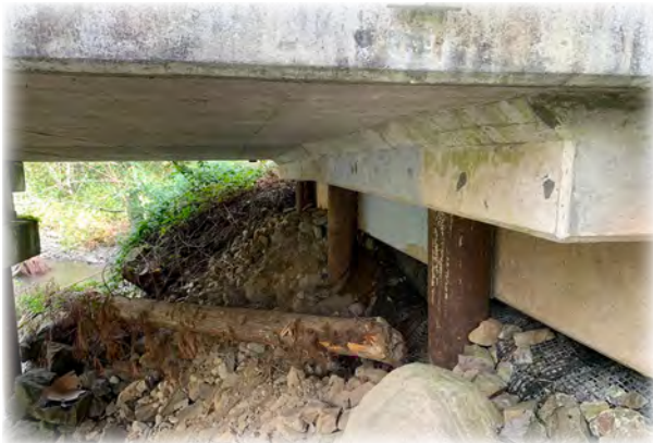
Wallace River Bridge 536 built in 1970 in Gold Bar. The rock abutment wall wrapped in geogrid at the south end of the bridge was punctured by a log during a highwater event causing the wraps to collapse and roadway pavement to settle.
