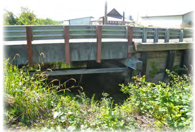
Portage Creek Bridge 311 on 43rd Ave NE in Arlington is a short span built in 1972. It's an example of one of our bridges that is a combination of wood and concrete construction.
