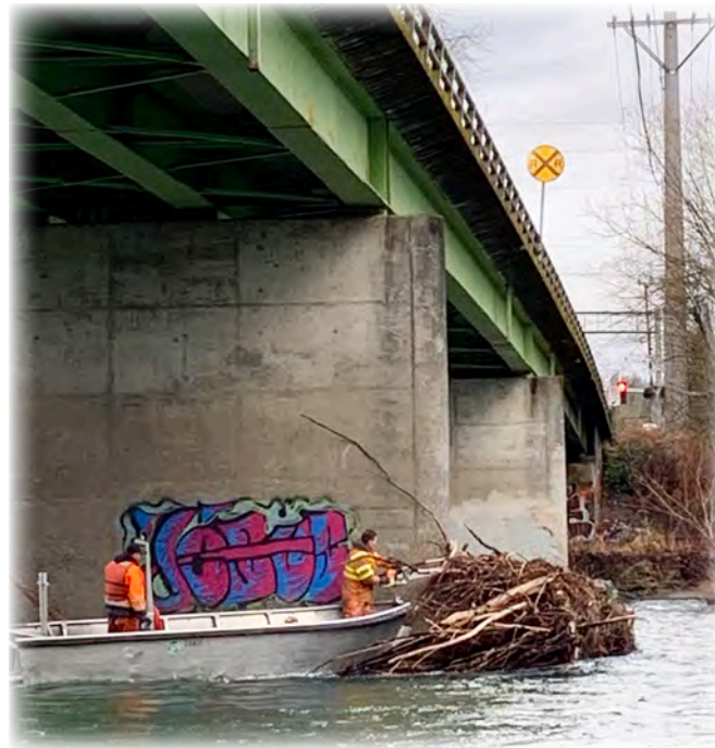
Sultan Bridge 94 on Mann Road and over the Skykomish River in Sultan was built in 1961. WSDOT maintenance crew members were hired by the county to break up some of the trapped wood debris at Pier 2.
