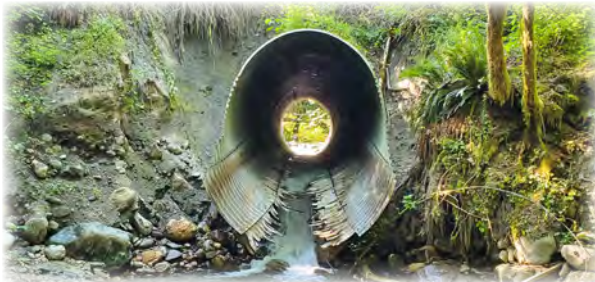
Metal culvert pipe damaged in early 2020.
