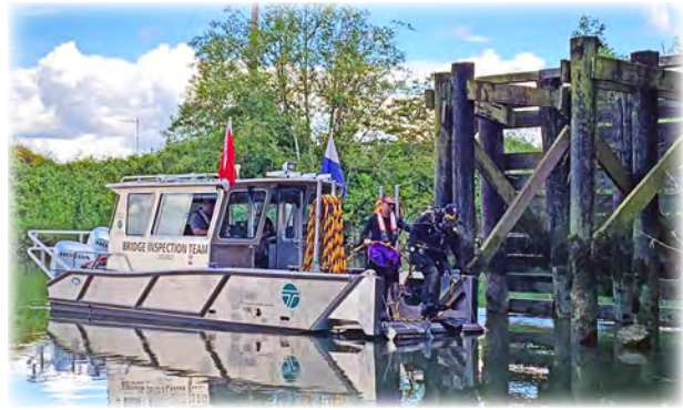
Ebey Slough Bridge 3 is one of five bridges which requires underwater inspections. Snohomish County works with the WSDOT underwater inspection diving team. Divers are checking scour depth.
