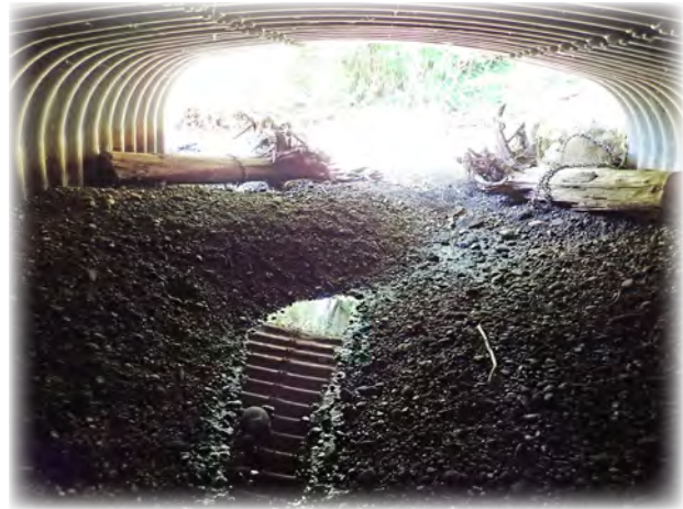
Bridge 14 is a corrugated aluminum culvert carrying Swamp Creek at the intersection of Gibson Road and Admiralty Way. A scour mitigation work order was completed in the fall of 2017.
