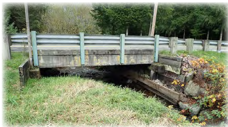
Barr Creek Bridge 158 is a short span bridge on Ben Howard Road and built in 1956 in the Monroe area. It is functionally obsolete due to its narrow deck width and high ADT, which classifies it as a future replacement candidate.
