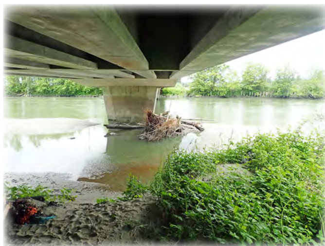
Jim Donner Bridge 4 with a log jam at one of the internal piers due to flood waters. Bridge was built over the Stillaguamish River on Marine Drive in 1985.
