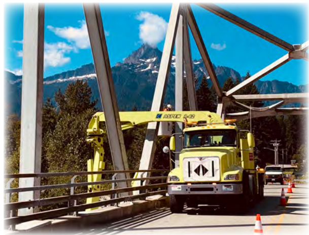
Sauk River Bridge 414 on Sauk Prairie Road. County and WSDOT bridge inspectors inspecting the bridge's steel truss via a WSDOT UBIT.
