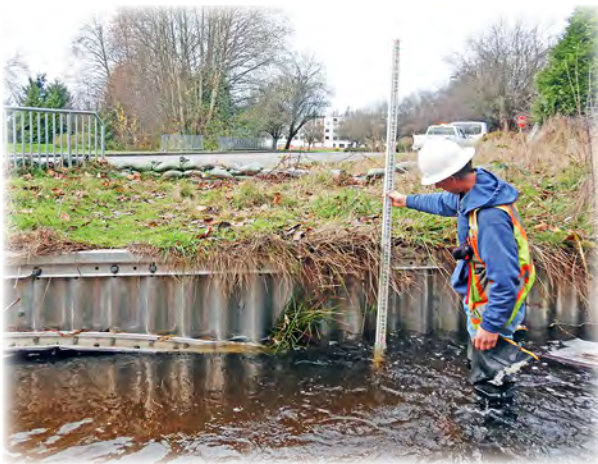
The inspector pictured above is measuring scour on Prairie Creek Culvert for the city of Arlington.
