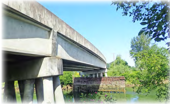
Ebey Slough Bridge 3 built in 1976 on Home Acres Road is one of the county's Lifeline Route bridges. It is located in Everett in the Snohomish River valley 1.3 miles east of Lowell and the Snohomish River.
