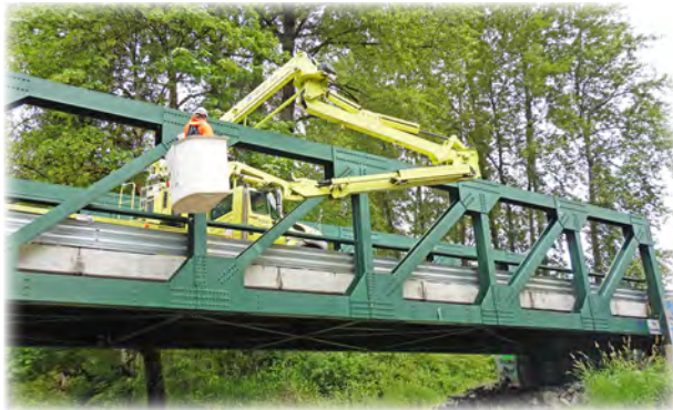
Pilchuck River Bridge 581, built in 2016 near Lochsloy, is one of nine steel trusses in the county. The bridge underwent a biennial special inspection in 2021 utilizing a WSDOT UBIT truck.
