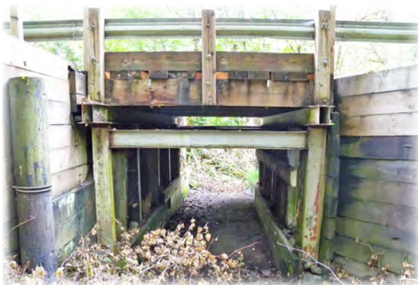
Everett Creek Bridge 565 located 3.5 miles northeast of Darrington on Crawford Loop Road was built in 1985. It is a short span with an overall length of 15 feet (NBIS length of 12 feet) and has a fish passage restriction. The bridge is planned to be replaced with a longer structure.
