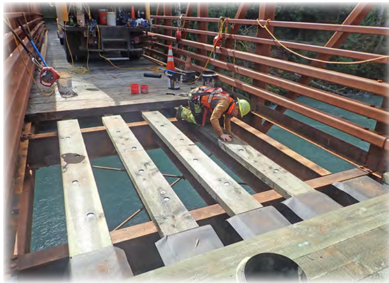
South Fork Stillaguamish Bridge 660 retrofit. The crew is attaching pressure-treated nailer planks to steel stringers for decking system replacement.
