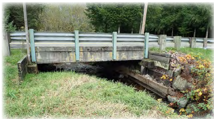
Barr Creek Bridge 158 is a short span bridge on Ben Howard Road and built in 1956 in the Monroe area. It is functionally obsolete due to its narrow deck width and high ADT, which classifies it as a future replacement candidate.
