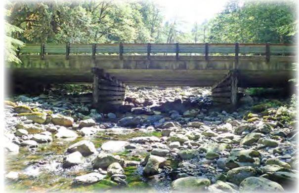
Black Creek Bridge 547 built in 1952 on Mountain Loop Highway. Exposure of shallow concrete spread footings classifies this scour critical bridge as a future rehabilitation candidate.
