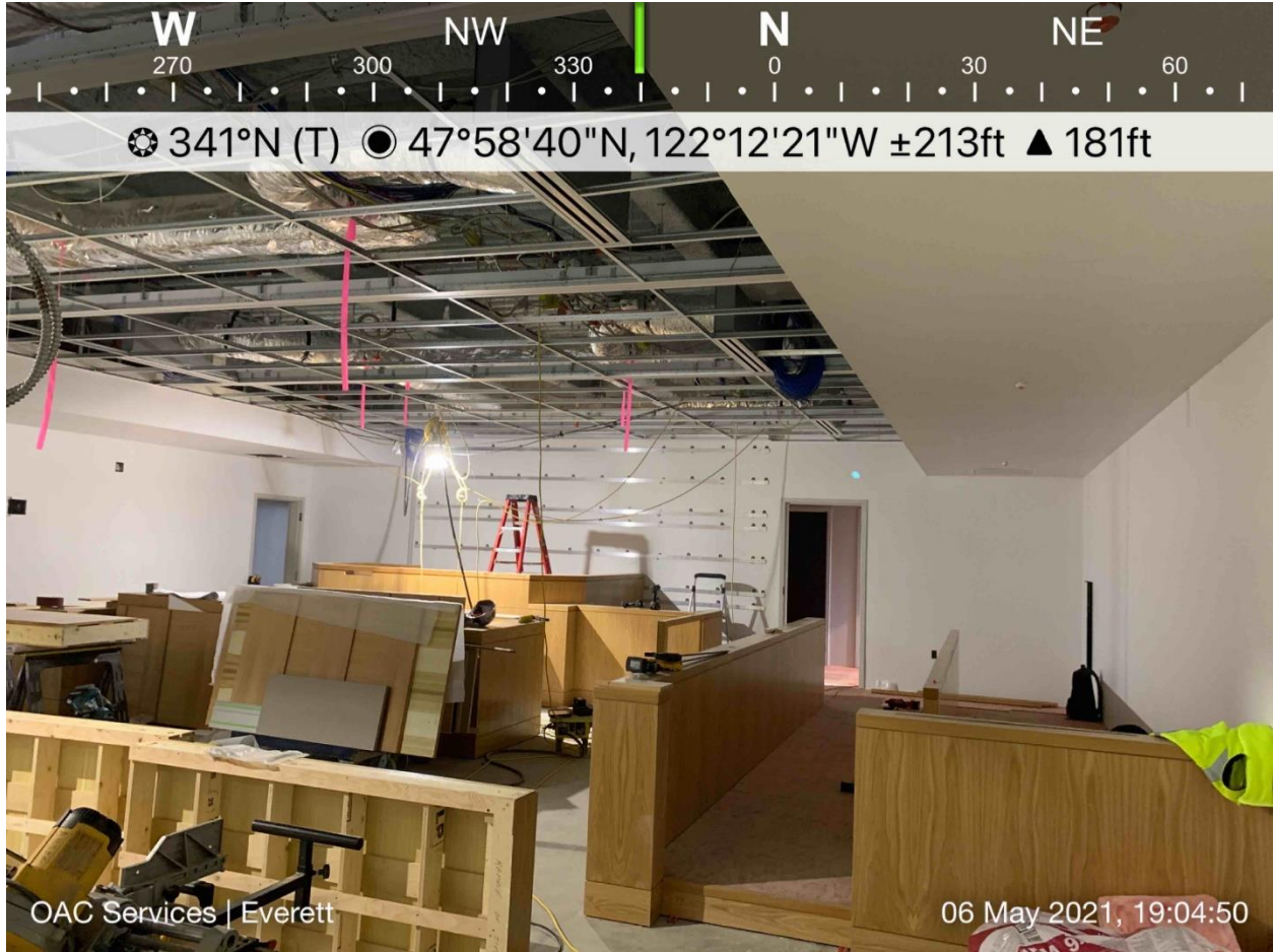
Courtroom 4A bench, jury box, and head wall construction progress in early May.
