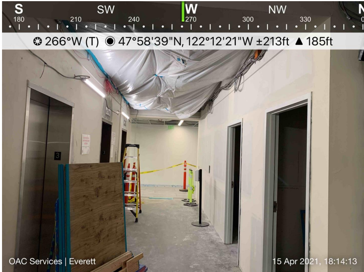
Third-floor elevator lobby in mid-April. View is east toward the District Court courtrooms.
