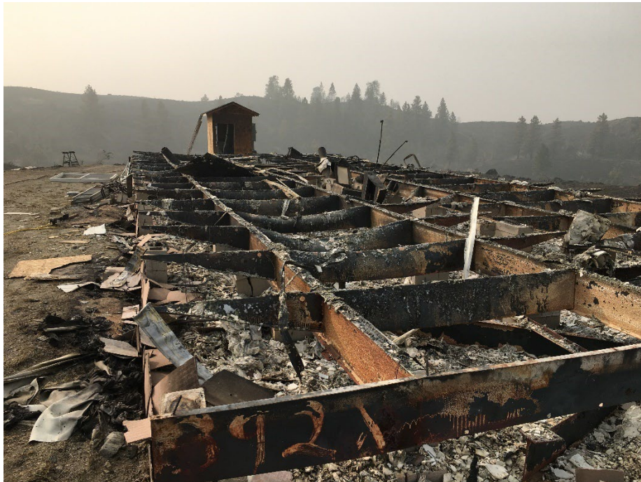
Figure 26 – A foundation lies in ruins after the Cold Creek Fire in Okanogan County in 2020.
