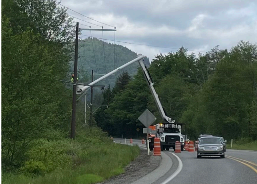
Figure 13 – A SnoPUD tree trimming contractor works on the Highway 530 corridor near Oso
