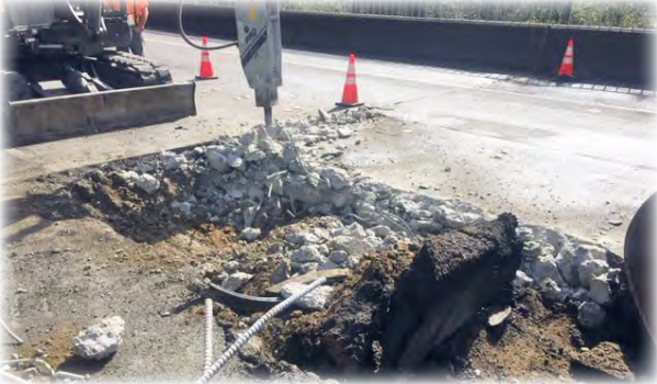
County Bridge Maintenance demolishing existing slab at the northwest corner of the bridge.
