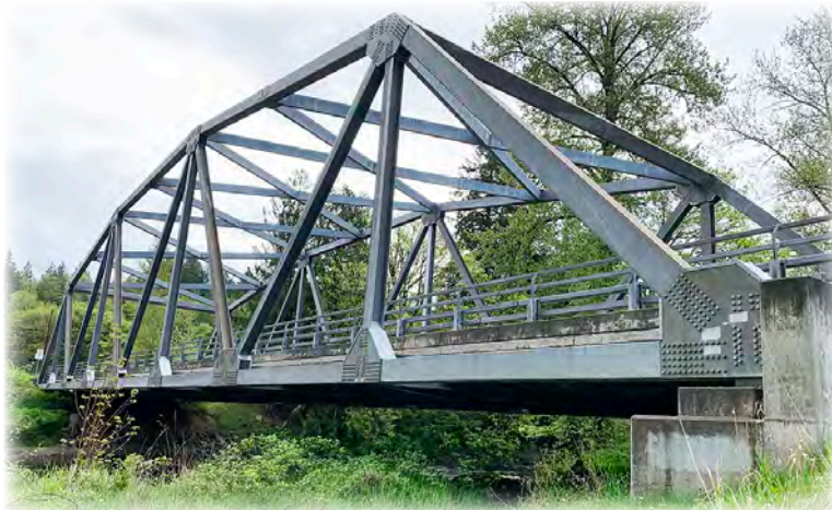
Machias-OK Bridge 44 over the Pilchuck River is one of nine steel trusses in the county and was built in 2005 on OK Mill Road in Snohomish. It is one of 11 fracture critical bridges in the county and it underwent a biennial special inspection in 2020.
