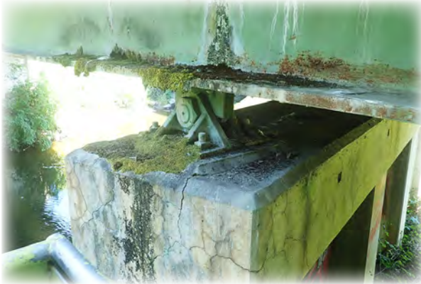
Pilchuck Creek Bridge 626 on Old 99 North and built in 1933. Rusting steel girders, exposed aggregate on concrete deck and significant cracking of many other concrete elements classifies this bridge as a future rehabilitation candidate.
