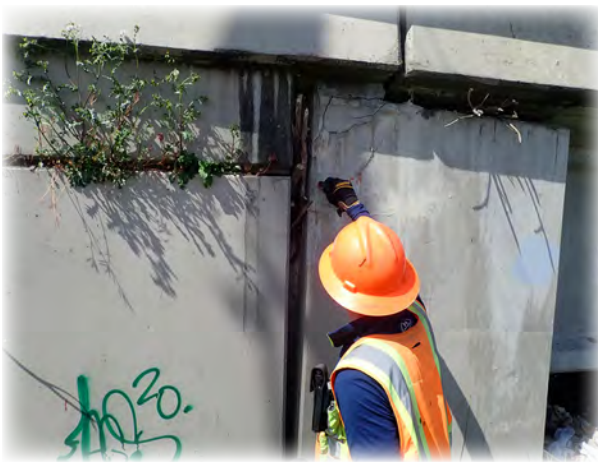
Snohomish River Bridge 1 on Airport Way in Snohomish. County inspector setting marker to monitor gap between mechanically stabilized earth (MSE) wall and Abutment 1.
