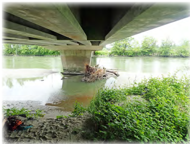
Jim Donner Bridge 4 with a log jam at one of the internal piers due to flood waters. Bridge was built over the Stillaguamish River on Marine Drive in 1985.
