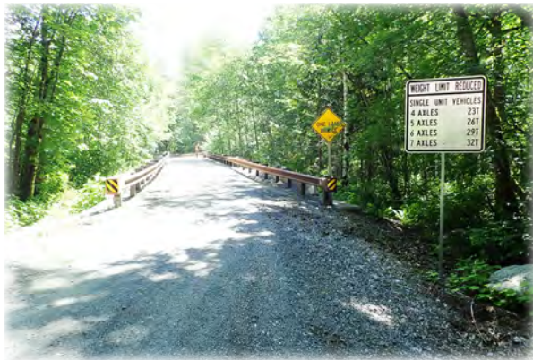
South Fork Sauk River Bridge 540 on Reece’s Hideout Road has a both a width and weight restriction.
