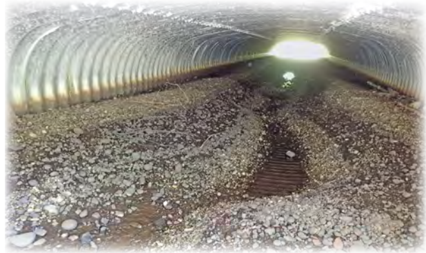
Bridge 14 (Culvert C14) carrying Swamp Creek at the intersection of Gibson Road and Admiralty Way. A work order is planned for 2021 to repair voids under the sidewalk located just upstream of the bridge.
