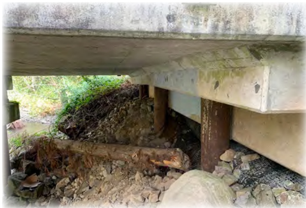
Wallace River Bridge 536 built in 1970 in Gold Bar. The rock abutment wall wrapped in geogrid at the south end of the bridge was punctured by a log during a highwater event causing the wraps to collapse and roadway pavement to settle.
