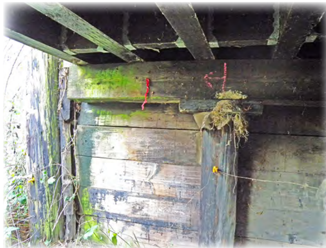
Miller Road Cattle Pass Bridge 116, a short span bridge built in 1963 and located south of Stanwood. It also serves as a flood relief channel for the adjoining valley. In 2021 one cap and four abutment boards will be replaced and three structural piles will be reinforced due to advanced to intermediate decay.
