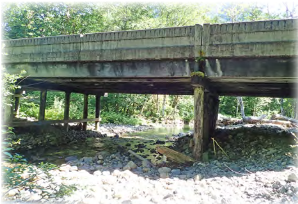
Deer Creek Bridge 670 built in 1949 on Mountain Loop Highway. Currently has 13 lines of 6 spans of original 8 x 24-inch treated timber sawn girders, and original concrete deck and railing.
