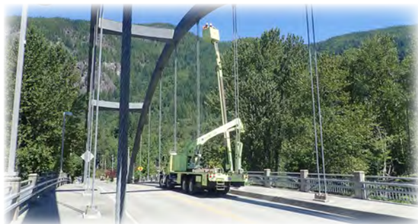
Wes Smith Bridge 122 over the N.F. Skykomish River in Index. County and WSDOT bridge inspectors inspecting the bridge’s steel arch and cables via a WSDOT UBIT.
