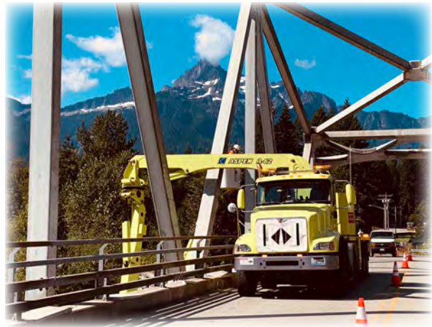
Sauk River Bridge 414 on Sauk Prairie Road. County and WSDOT bridge inspectors inspecting the bridge's steel truss via a WSDOT UBIT.
