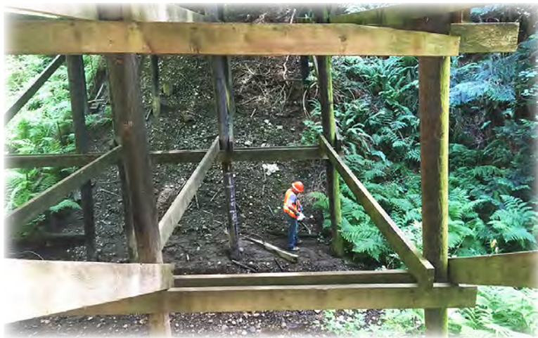
Fisher Creek Bridge 433 on English Grade Road. County bridge inspector examining timber piles and braces.
