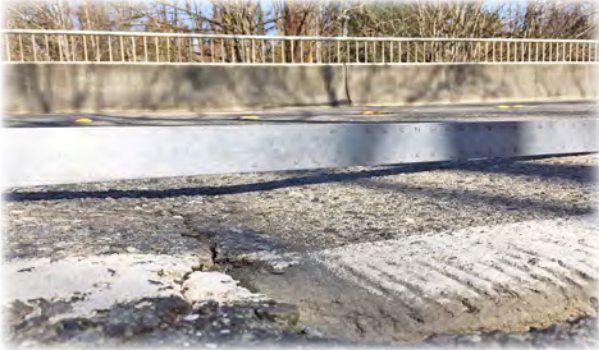
Straight edge shows abrupt dip at connection between concrete approach slab and asphalt roadway.
