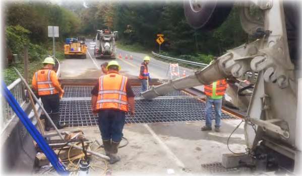
County Bridge Maintenance preparing to pour the new slab at the northeast corner of the bridge.
