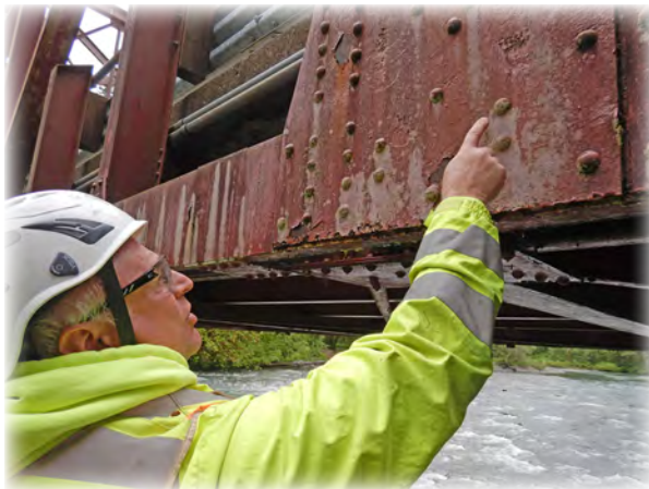
Red Bridge 537 undergoes a required Fracture Critical Inspection every 24 months. All members of the steel truss bridge are carefully inspected for signs of stress and fatigue.
