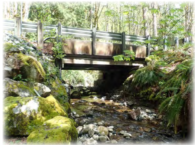
Hogarty Creek Bridge 636 on Reiter Rd in Sultan is a short span built in 1997. It’s an example of one of our bridges that is a combination of wood and concrete construction.
