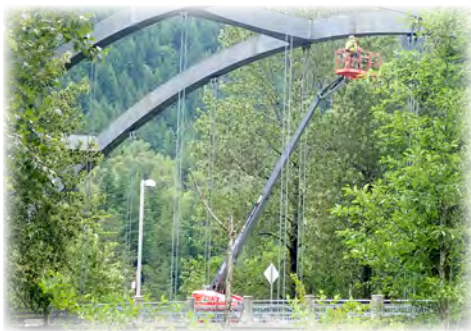
Wes Smith Bridge 122 over the N.F. Skykomish River in Index. WSDOT inspectors are inspecting the bridge's steel arch and cables from a boom lift.
