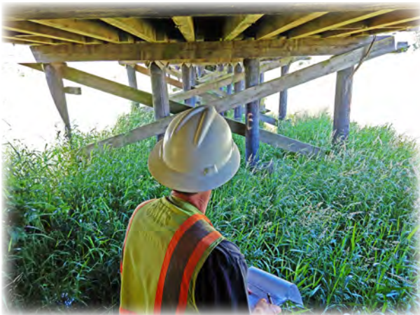
Norman Slough Bridge 430 on Olson Rd. County bridge inspector is evaluating the condition of the timber members.
