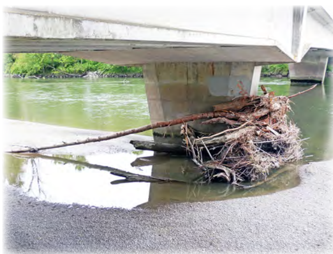
Jim Donner Bridge 4 with a log jam at one of the internal piers due to flood waters. The bridge was built over the Stillaguamish River on Marine Drive in 1985.
