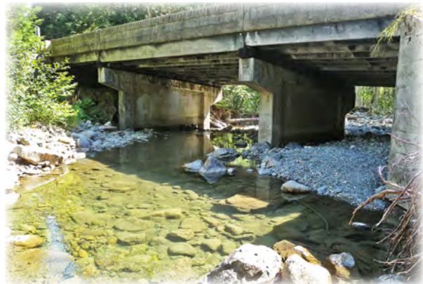
Coal Creek Bridge 556 built in 1949 on Mountain Loop Highway has original 6 x 20-inch (spans 1 and 3) and 8 x 24-inch (span 2) treated timber sawn girders, and original cast-in-place concrete piers, deck and railing.
