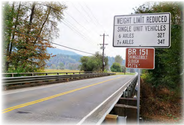
Shinglebolt Slough Bridge 151 on 311th Ave SE has new weight limits posted restricting larger trucks with six or more axles.
