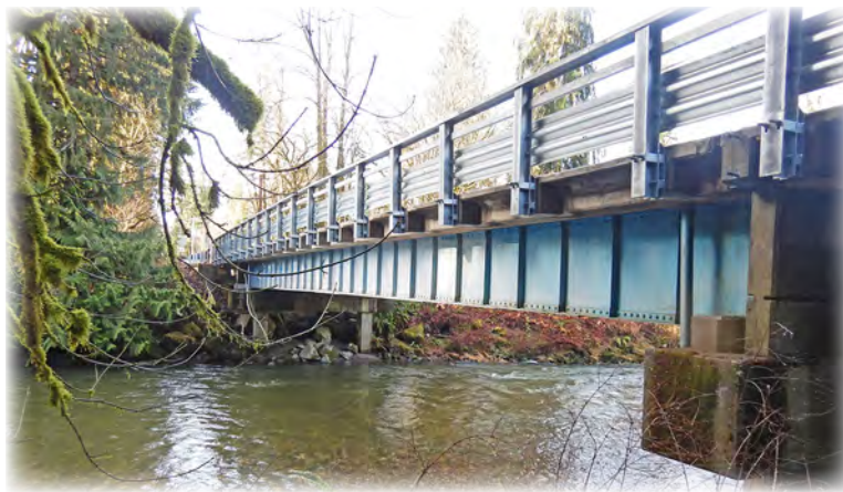
The 2022 rehabilitation package for Madden Bridge 58 included a new concrete deck, bridge rail, bearings, and guardrail approaching the structure. The bridge was built in 1956 and carries Menzel Lake Rd across the Pilchuck River.
