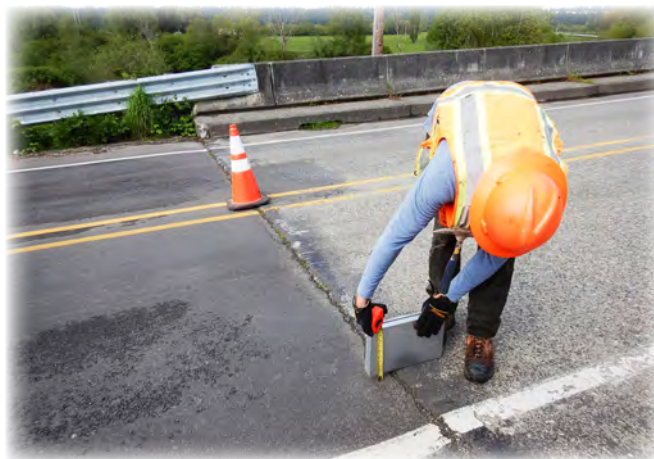
Ebey Slough Bridge 3 on Home Acres Rd. County bridge inspector is measuring settlement of the approach roadway.
