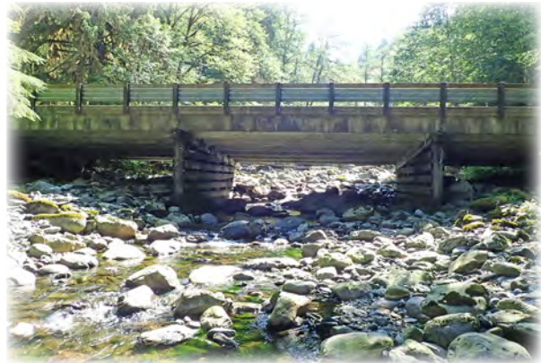
Black Creek Bridge 547 built in 1952 on Mountain Loop Highway. Exposure of shallow concrete spread footings classifies this scour critical bridge as a future rehabilitation candidate.
