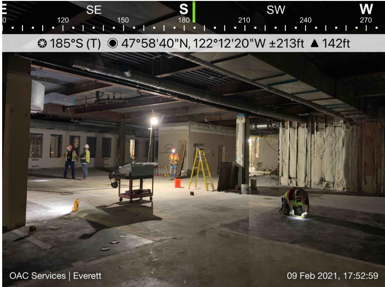
Future Superior Court Courtroom 4A in early February, looking southwest across the bench area from the jury deliberation room toward the elevator bank and the defendant table.
