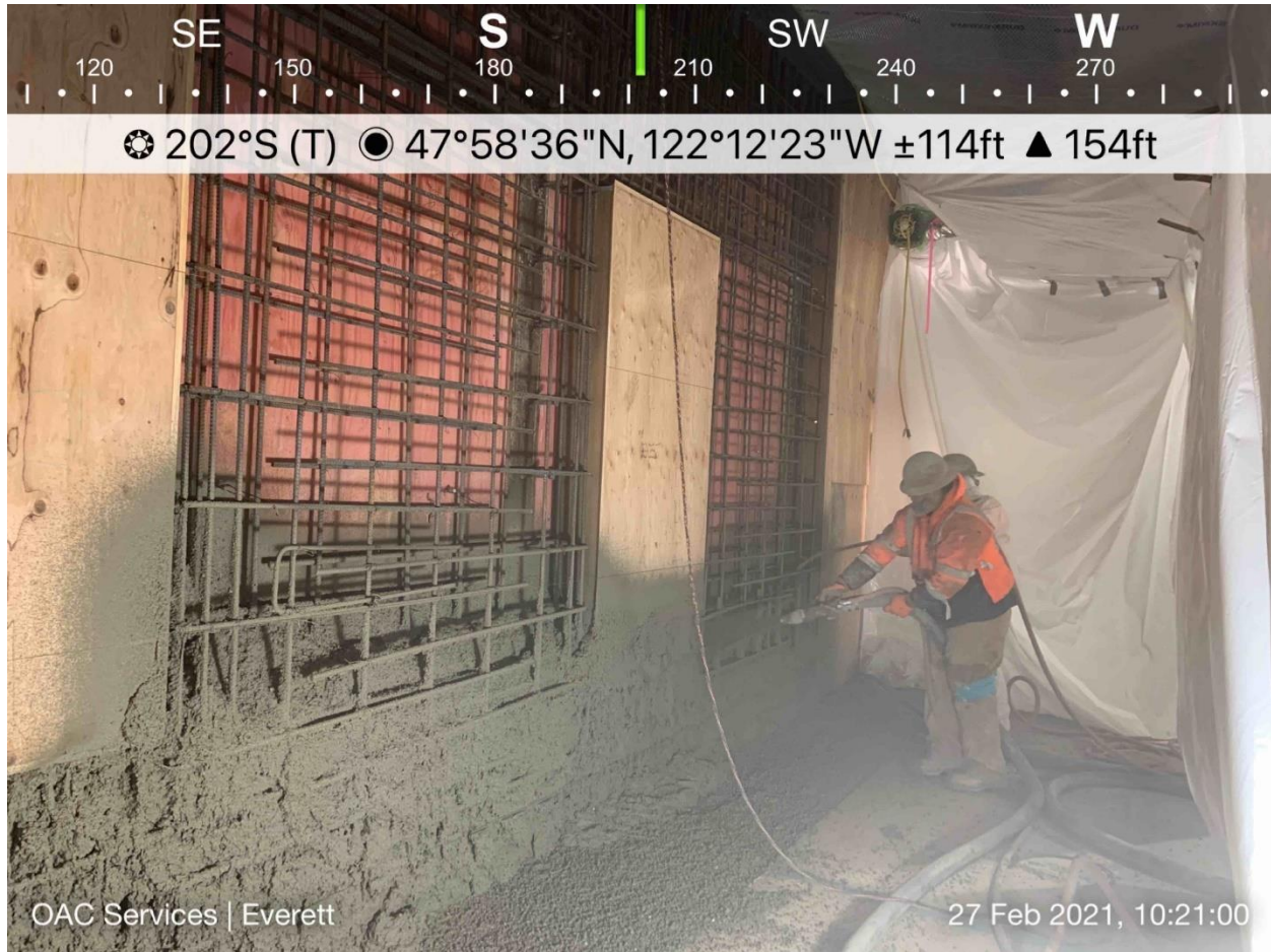
Shooting concrete for the Level 4 segment of the shearwall. Crews shot concrete for the shearwall on two consecutive Saturdays, three floors at a time from Basement to Level 5.
