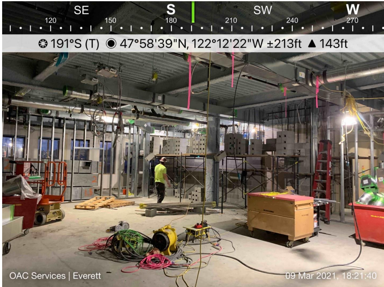
Superior Court Courtroom 4A one month later. Wall framing in the left and center background would be at the back of the gallery and for the public access corridor.
