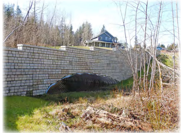
Reiner Bluff 675 is a developer-built corrugated steel arch culvert spanning 54 feet over a wetland on 120th St. SE just northwest of Sultan.
