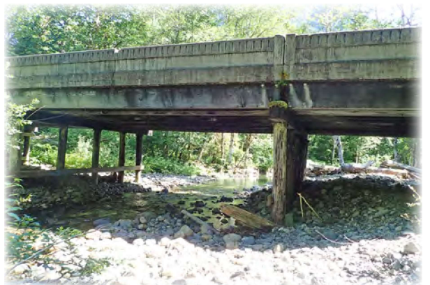
Deer Creek Bridge 670 built in 1949 on Mountain Loop Highway has original 8 x 24-inch treated timber sawn girders, and original concrete deck and railing. The bridge was retrofitted in 2023.
