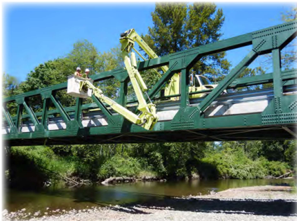
County and WSDOT Inspectors in UBIT conducting the NSTM inspection on Pilchuck River Bridge 581. All steel tension members are required to be inspected at hands length.
