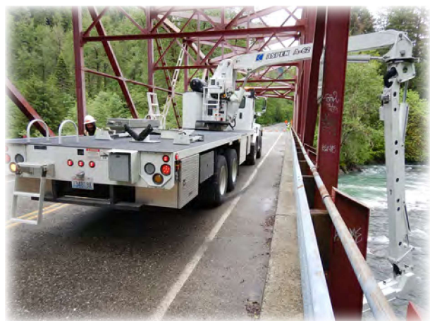
Red Bridge 537 on the Mountain Loop Highway. County and WSDOT inspectors are inspecting the bridge's steel truss via a WSDOT UBIT.
