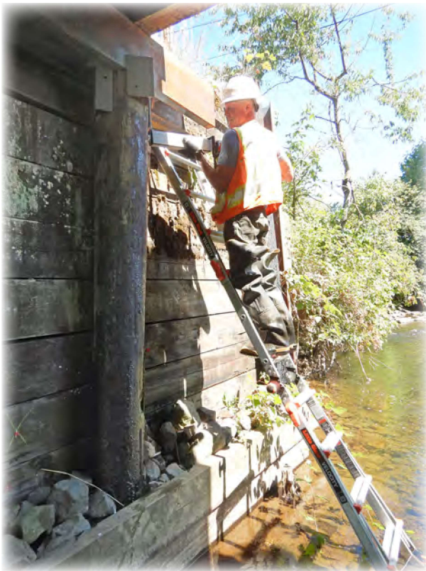
County bridge inspector drilling a timber pile at Bridge 443 to evaluate the condition and detect any decay.
