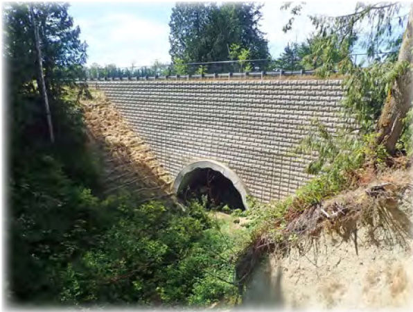
Woods Creek Vista B 682 is a developer-built corrugated steel arch culvert spanning 32 feet over an unnamed creek in a new housing development just northeast of Monroe.
