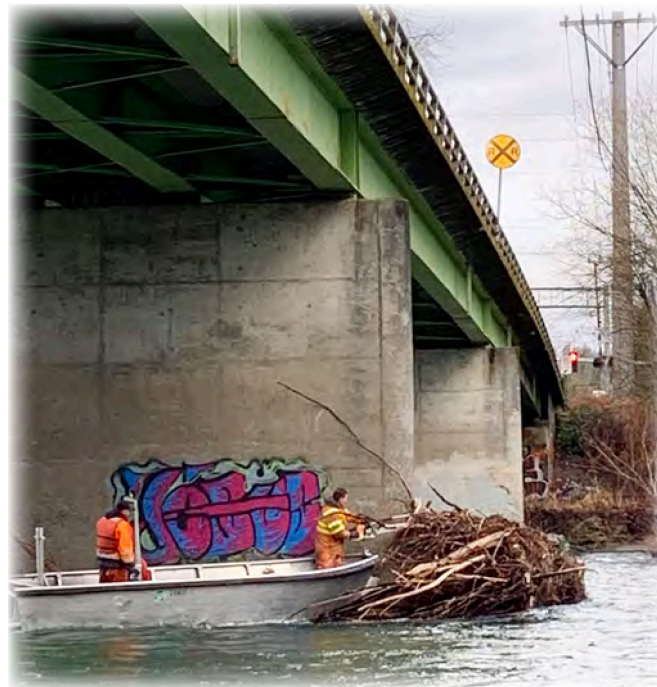
Sultan Bridge 94 on Mann Road and over the Skykomish River in Sultan was built in 1961. WSDOT maintenance crew members were hired by the county to break up some of the trapped wood debris at Pier 2.
