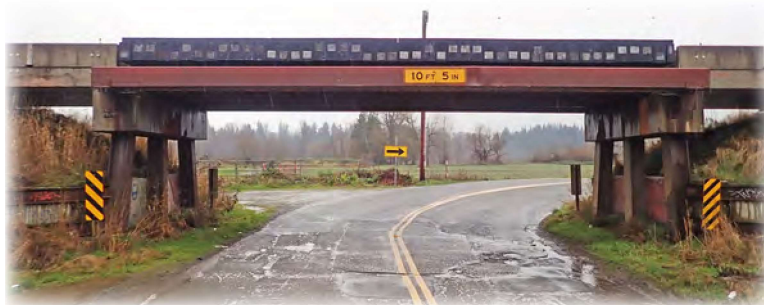
Norman Road Underpass is height restricted. Snohomish County conducts a Safety Inspection of this BNSF steel and concrete bridge constructed in 2013 near Stanwood.
