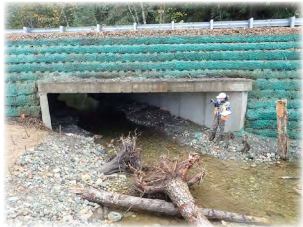
County bridge inspector performing the initial inspection of a new culvert on Mann Road.
