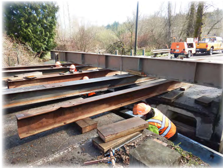
Snohomish County Bridge Crew jacking up Bear Creek Bridge 625 for replacement of the rotten timber caps.
