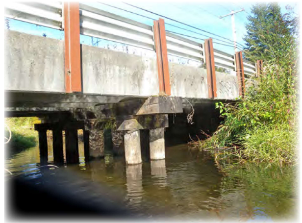
Gregory Road Bridge 272 is a two span bridge built in 1961. The bridge has a concrete tub superstructure and timber substructure. The condition of the substructure needs extensive maintenance and repairs and warrants a Structurally Deficient status. The county will pursue replacement funding.
