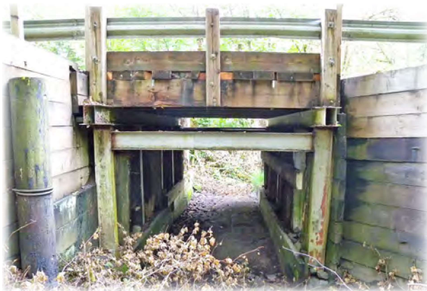
Everett Creek Bridge 565 located 3.5 miles northeast of Darrington on Crawford Loop Road was built in 1985. It is a short span with an overall length of 15 feet (NBIS length of 12 feet).
