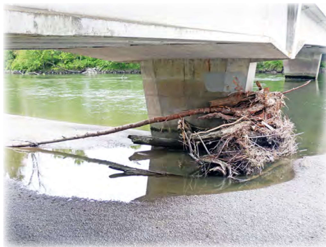
Jim Donner Bridge 4 with a log jam at one of the internal piers due to flood waters. The bridge was built over the Stillaguamish River on Marine Drive in 1985.
