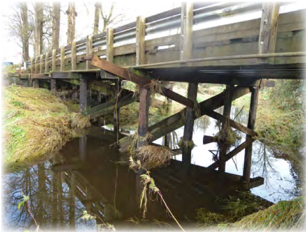
Riley Slough Bridge 52 is a four span bridge built in 1970. The bridge has a timber deck, superstructure, and substructure. Extensive repairs to the bridge necessitated a full road closure, and the condition of the substructure warrants a Structurally Deficient status. The county will pursue replacement funding.
