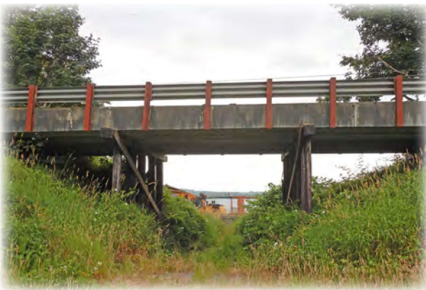
Cattle Pass Bridge 183 is a three span bridge on Lowell-Larimer Road, which was last rebuilt in 1966. The deteriorating wood substructure necessitated a load posting in 2023. The bridge is on an important agricultural and commuter route, as well as a seismic lifeline route. The county will pursue replacement funding.
