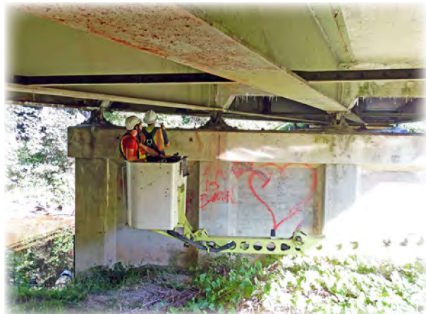
Pilchuck Creek Bridge 626, built in 1933, requires a Special Feature Inspection of the steel pins every 72 months. Ultrasonic Testing (UT) equipment provides an effective, non-destructive method to assess the condition of steel members.
