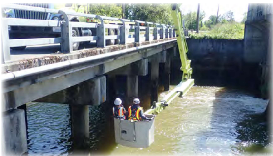
County and WSDOT inspectors looking at the girders and substructures of a City of Everett bridge from the UBIT.
